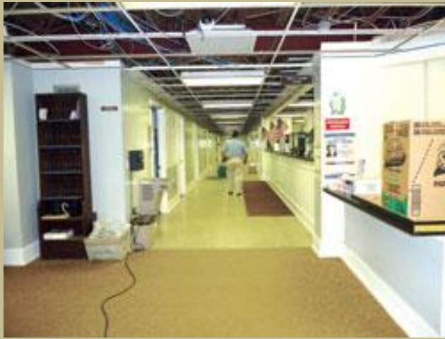
1 st floor scene – County Office Building after fire, ceiling tiles removed.
